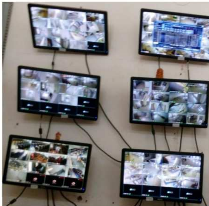
CCTV Control Room
